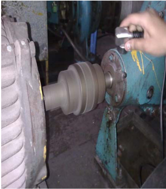
Fig. 1 Motor Pump Assembly.
